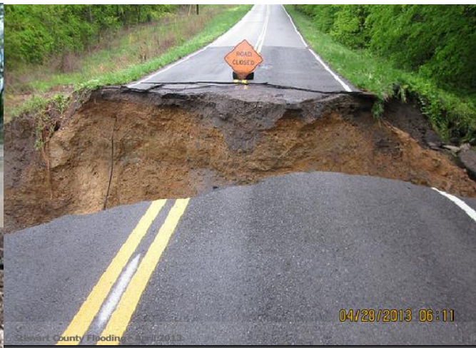
Stewart County Flooding April 2013
